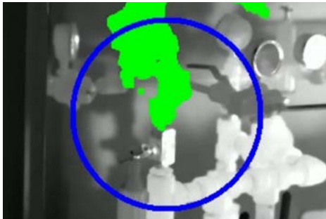
Quantifies gas, such as the methane escaping this wellhead valve at 0.59 lb/hr
