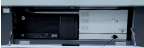
PC, controller unit storage
